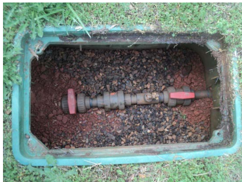
Inside Low Pressure Sewer Box
