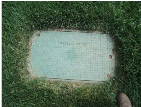
Low Pressure Sewer Box
